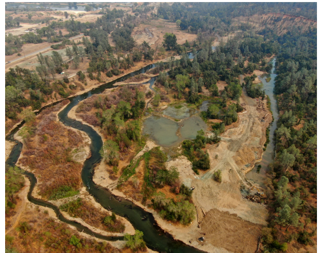
A new stream channel created during the final stage of the Lower Clear Creek Floodway Rehabilitation Project provides islands, riffles, side channels and alcoves that improve fish habitat and fish passage. Credit: Aaron Martin/ Yurok Tribe Design Team
