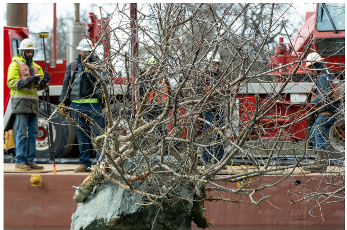
Rockwads project to provide deep-water rearing habitat for juvenile salmonids on the Sacramento River. Photo courtesy of the Sacramento River Settlement Contractors.
