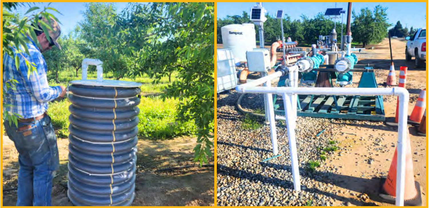
Left: Robert Wilmott (orchard manager) looking over the reverse tile drain system on Fresno State almond field. Right: Filter and pipeline delivery for the system.
